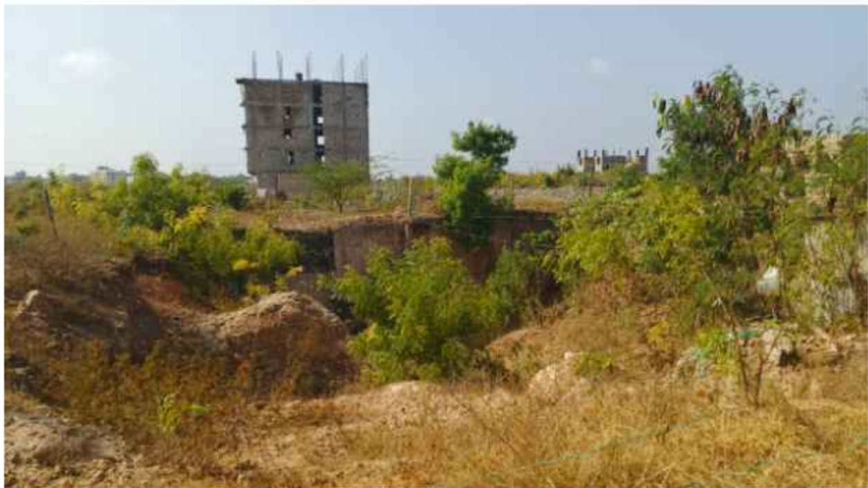
FIGURE 4: Ongoing constructions in clear disregard to the 2023 court order
